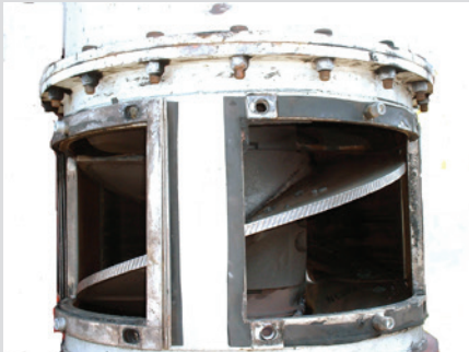
OD bearing house with removed covers
