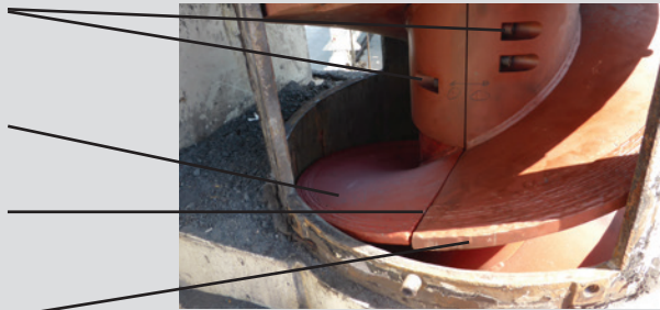
Inside the OD bearing house
